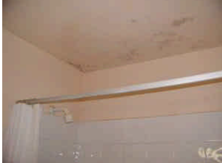
Mould growth on ceiling of poorly ventilated hotel bathroom
