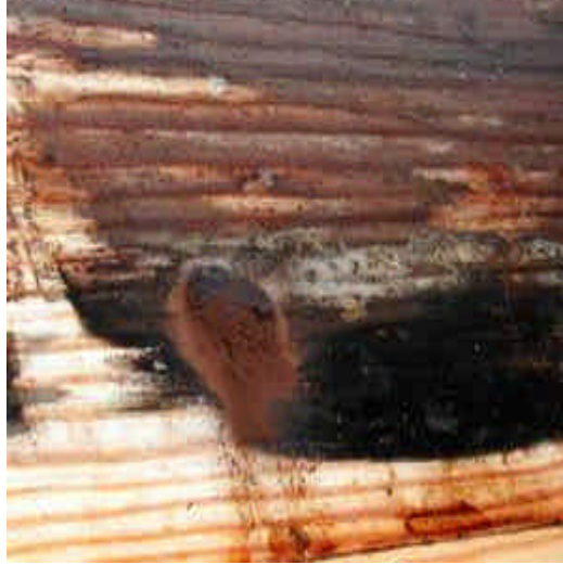
Close-up of mould growing on wood
