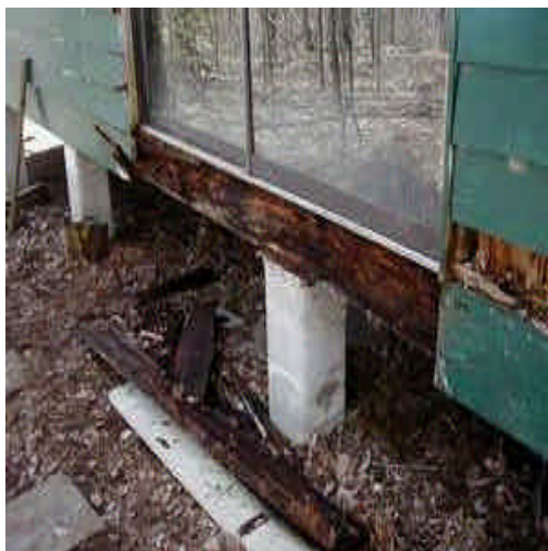
Decay fungi attacked the perimeter wood beam where rain water leaked in around the patio door
