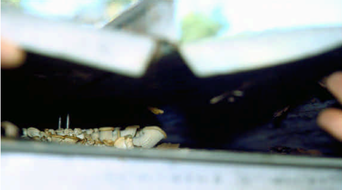
Mushrooms can be seen growing on the wood substrate, fed by water leaking through a standing seam roof (out of focus, above)
