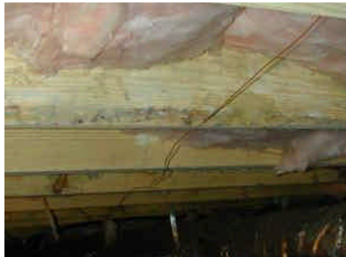
These 3 month old crawlspace joists were kept cool (18 °C) by the soil resulting in high humidity and condensation when warm humid summer air from outdoors entered through vents
