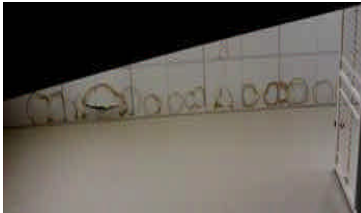
Air leakage condensation from an adjoining pool caused wetting and consequent staining and mould growth on the ceiling tiles of this stairwell next to an interior wall of this school
