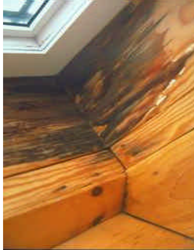
Rain leaking through the skylight in this bathroom caused mould growth on the wood trim
